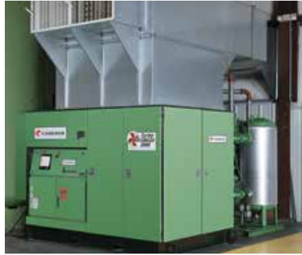
112 kW (150 hp) TURBO-AIR Cooled and TURBO DryPak compressors installed at a manufacturing plant, hot air from air coolers are used to heat the factory.
