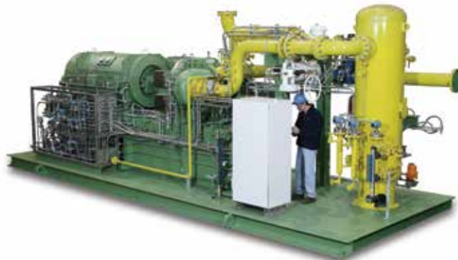
Fuel gas booster skid
