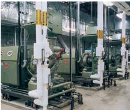
Three 150 kW (200 hp) TURBO-AIR compressors installed at an electronics facility.
