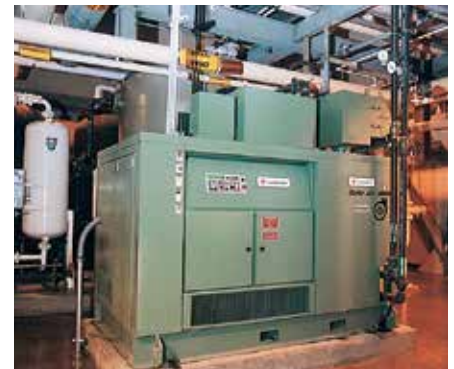
One 225 kW (300 hp) TURBO-AIR compressor installed at a major university for instrument air.
