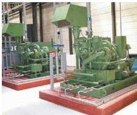
260 kW (350 hp) TURBO-AIR compressors installed at an automotive facility.
