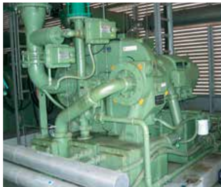
225 kW (300 hp) TURBO-AIR compressor installed at a semiconductor facility.
